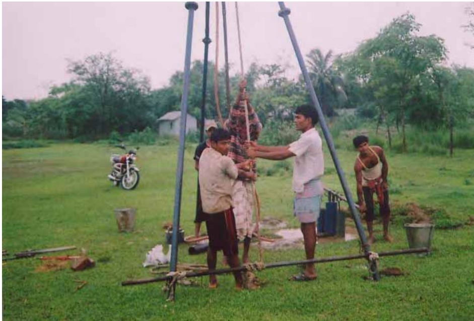
Photograph of field Boring and SPT Sample of Bore Hole – 08 in field
