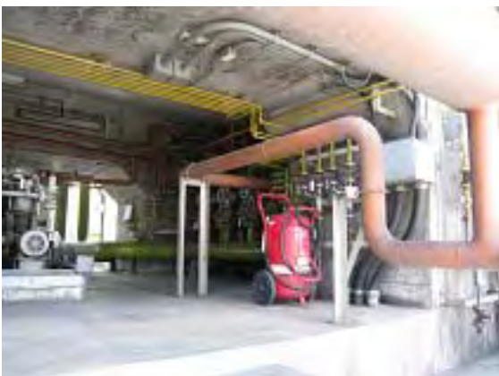
Equipped with firefighting equipment
