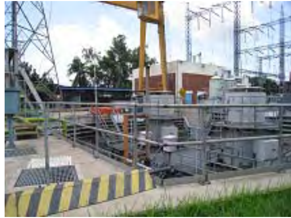
Equipped with safety fences (for fall prevention)
