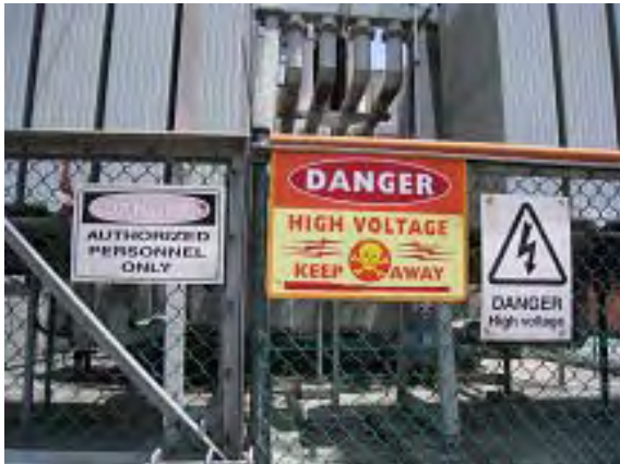
Safety signs (Significantly dangerous spot: Keep away from high voltage)
