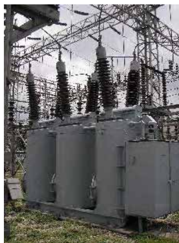
Figure I-5-5-6 132kV substation OCB (1982)
