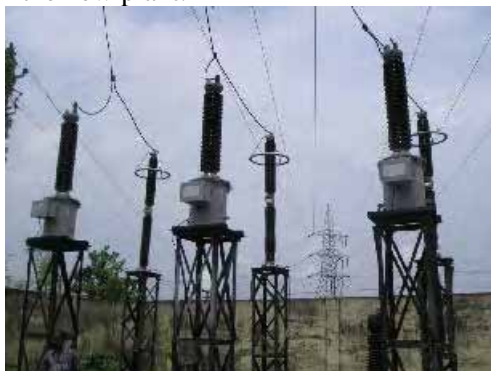
Figure I-5-5-4 VCT and LA of 132kV substation after replacement
