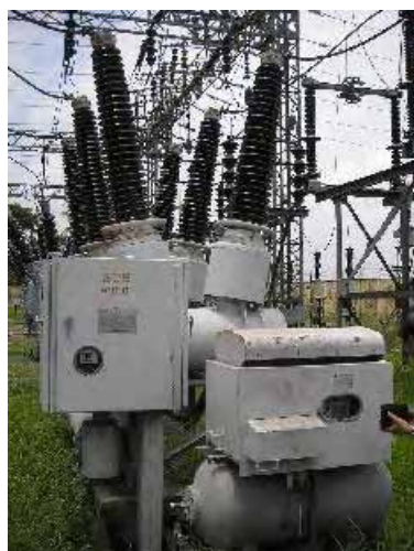
Figure I-5-5-5 132kV substation GCB (1979)
