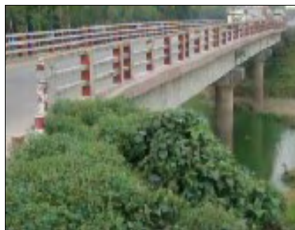
Photograph I-4-8-6 Weak RCC Bridge at 20 km from Sirajganj
