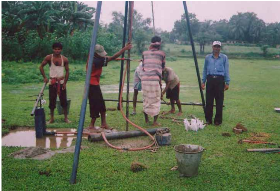
Photograph of field Boring and SPT Sample of Bore Hole – 05 in field
