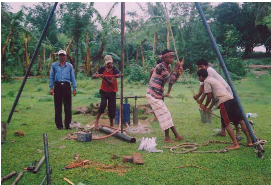
Photograph of field Boring and SPT Sample of Bore Hole – 06 in field
