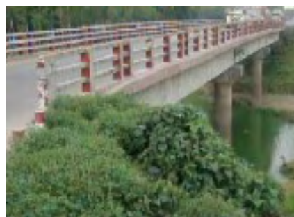
Photograph I-4-8-6 Weak RCC Bridge at 20 km from Sirajganj
