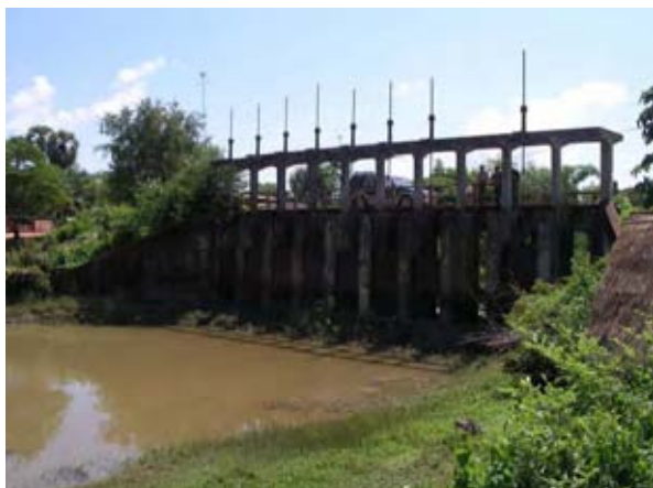
Existing Ream Kon Headworks not Functioning (Ream Kon Rehabilitation Sub-Project) (May 25th 2008)
