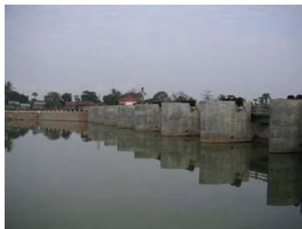
Existing Damanak Ampil Headworks Originally Constructed by MOWRAM in 2006 (Damanak Ampil Rehabilitation Sub-Project) (February 2nd 2008)
