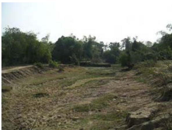
Existing Headworks, already Deteriorated and Not Functioned (Wat Chre Rehabilitation Sub-Project) (February 5th 2008)
