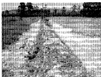
Bund Observed as Demarcation , but No Tertiary Canals Developed at Present (January 29 th , 2008)
