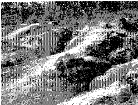
Severe Gully Erosion Due to Dispersive Sandy Soil in the Command Area (January 29 th 2008)
