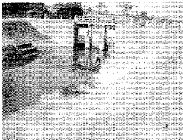
Check Gate on the Main Canal Constructed by MOWRAM in 2006 (February 2 nd 2008)
