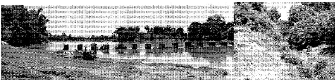
1. Ruins of pier of headworks in the Pursat River 2. Inlet of Wat Loung Main Canal
