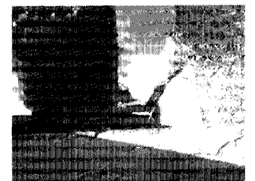
2. Crack of wing wall of intake
