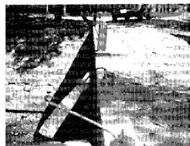
5. Broken handrail of bridge
