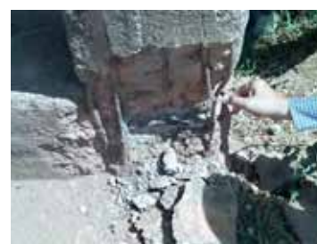
1. Damaged concrete and reinforcing bars exposed
