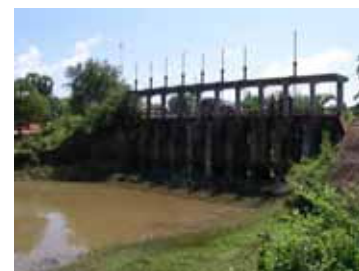
Existing Weir not Functioning (May 28 th , 2007)
