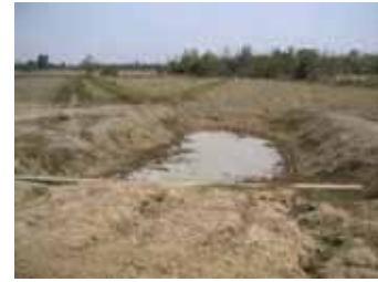
Outlet of Diversion Structure with no Secondary Canal Constructed (February 2 nd , 2008)
