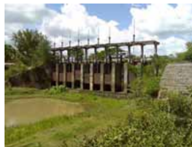
1. Upstream view of existing weir Gate lost function
