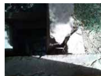
2. Crack of wing wall of intake
