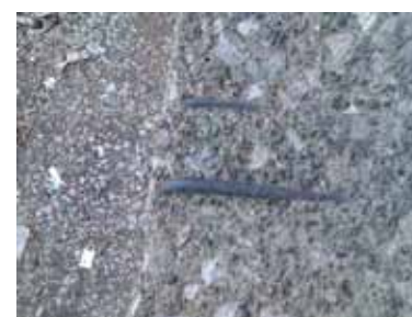
4. Exposed reinforcing bars
