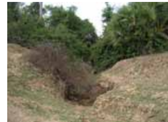
Beginning Point of Main Canal, since no Headworks, water inflows only in the flood period (February 2 nd , 2008)
