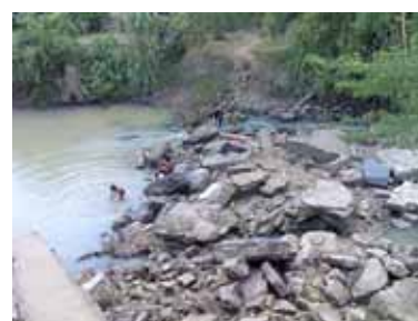
2. Broken diversion facility
