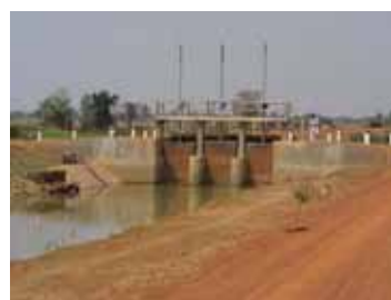
2. Check Structure on Main Canal
