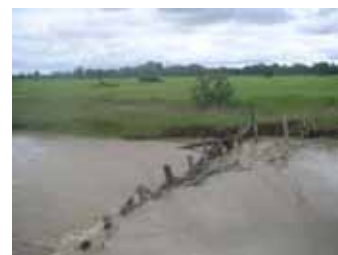
Main Canal with no Permanent Structures, Water Diverted using Wood Check (June 12 th , 2008)
