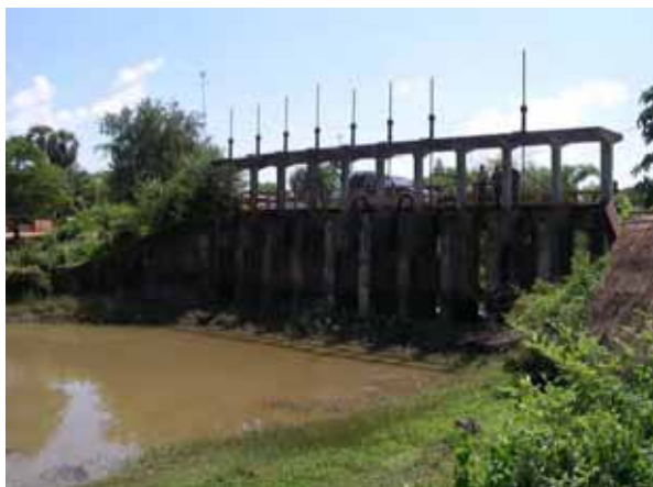
Existing Ream Kon Headworks not Functioning (Ream Kon Rehabilitation Sub-Project) (May 25th 2008)
