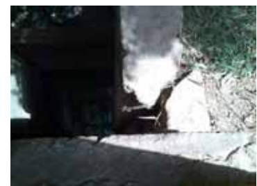
Cracks of Wing Wall of Intake (Por Canal Rehabilitation Sub-Project)
