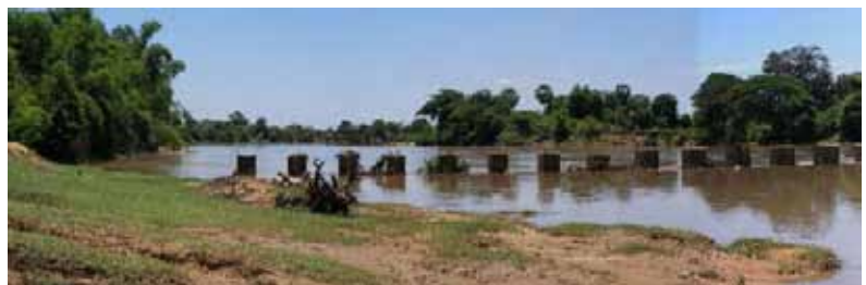
Ruins of Pier of Headworks on the Pursat River (Wat Loung Rehabilitation Sub-Project)
