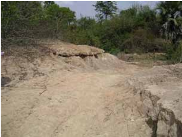
Main Canal Section, severely Deteriorated (Wat Loung Rehabilitation Sub-Project) (February 2nd 2008)
