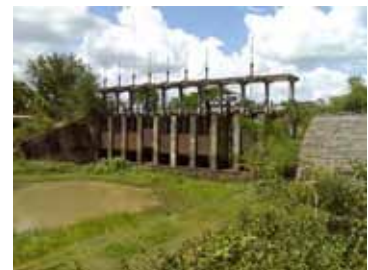
Upstream Feature of Headworks, Gate with no functioning (Ream Kon Rehabilitation Sub-Project)
