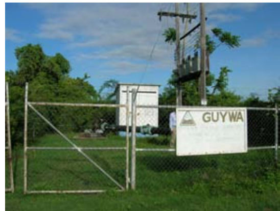
Existing Spring Garden pumping station. This well is a water source of the Queenstown WTP.
