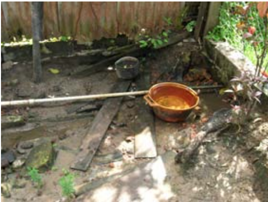
Low pressure water supply. Residents of this house can receive water only from this hydrant set at ground level.
