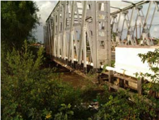
River crossing of the existing distribution trunk by bridge suspension
