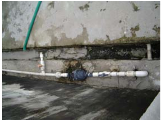
Exposed water meter. Service pipe is exposed and there is no cover of meter.
