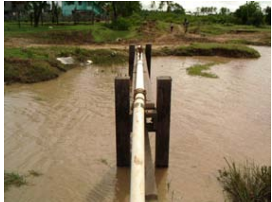
River crossing by wooden pile. Locally available hard wooden pile is resistant to corrosion. River crossing by wooden pile is common works in GWI.
