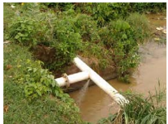
Leakage from distribution pipe. Possible damage by being exposed.
