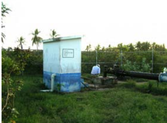
Existing No.57 Village pumping station. This well is a water source of the No.56 Village WTP. (Phase 1/2)
