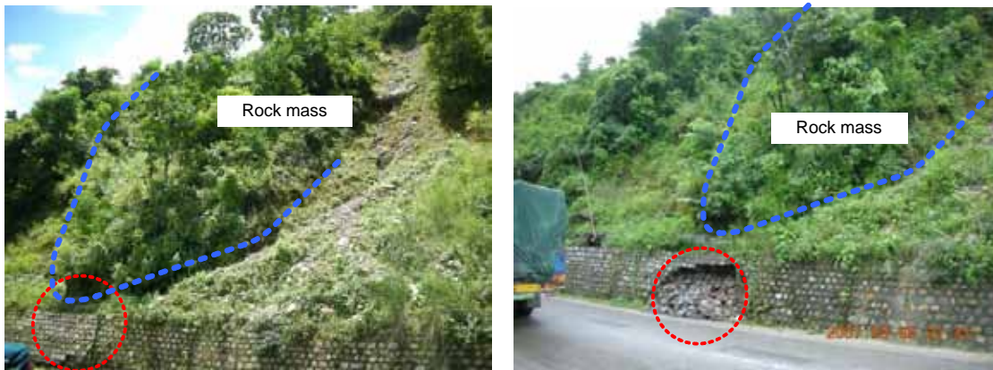
Figure 4.3.7 (a) Comparative photographs of a part of SL-3 slope (Right: Photo on August 2, 2007; Left: Photo on September 6, 2007)
