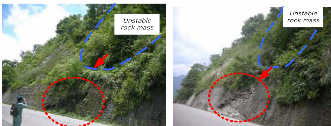
Figure 4.3.5 Comparative photographs of the masonry wall at SL-2. (right: photo on August 2, 2007; left: October 8, 2007)
