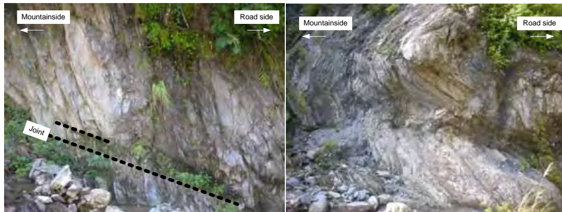
Figure 3.1.13 Non-tectonic deformations of phyllites of the Nourpul Formation (Left: road side-dipping joints, Right: gravitational fold of phyllites)
