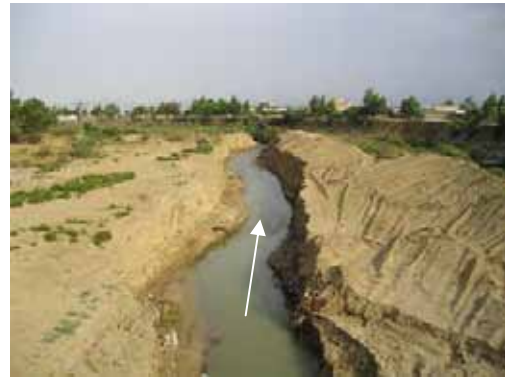
Downstream view from Bou Salem Bridge (A low water channel was constructed)
