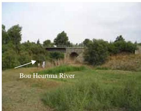
A view from upstream of Bou Heurtma Railway Bridge (heavy vegetation and narrow section)
