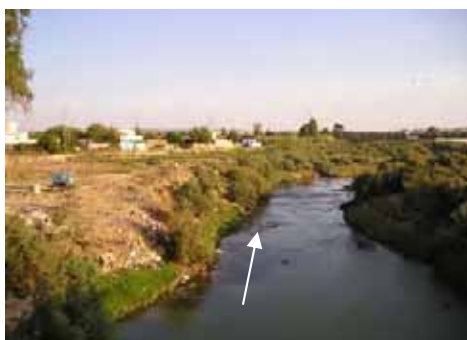
Downstream view from Jedeida Old Bridge (thick vegetation and heavy siltation can be seen at both banks)
