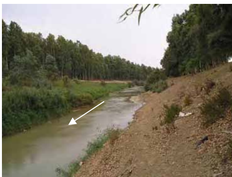
Upstream view of Jendouba Bridge (heavy siltation and narrow section by bridge structure)
