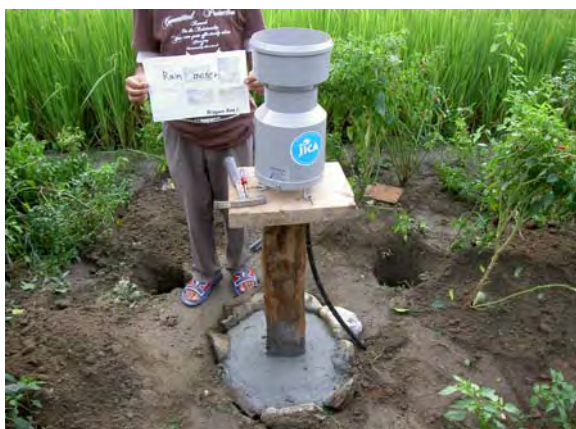
Installation completion of the rain gauge 1
