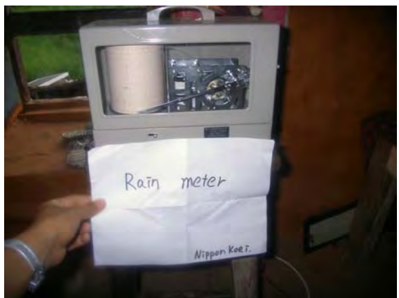
Installation completion of the rain gauge 4
