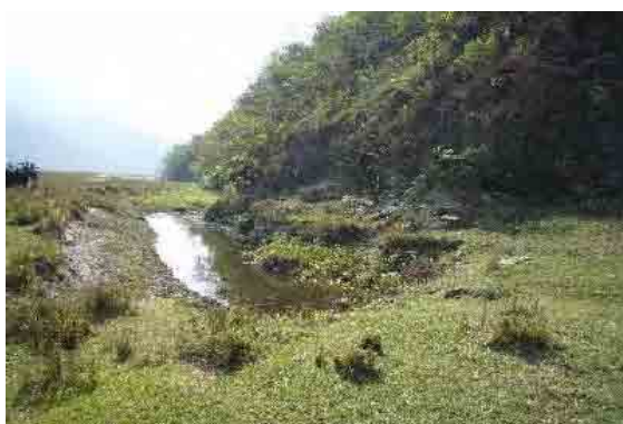
Photo 2-1 Scoring at CH27000 (3m)
