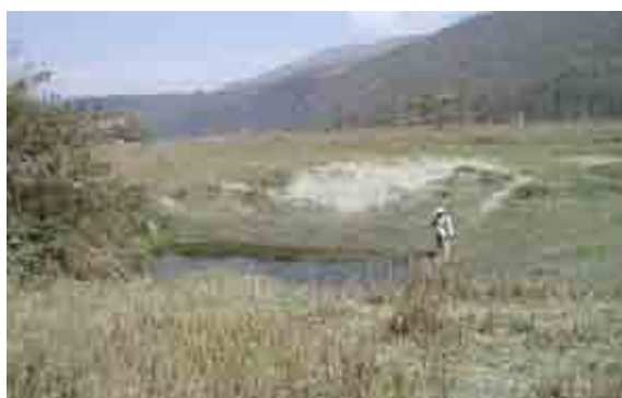
Photo 2-2 Scouring at CH27500 (4m)
