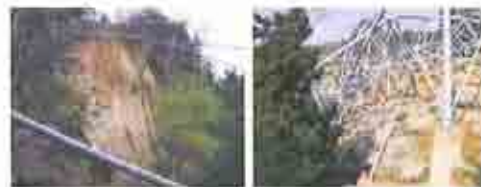
Tertiary landslide Left: crown, Right: destroy a steel tower (a pylon)
