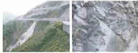
STA17 Failure of Rock
