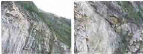
Sta17+ Loosed rock around Joint.
