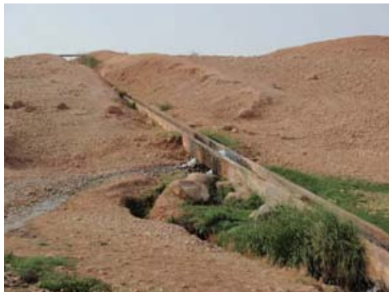
Leakage from spring water conveyance system
