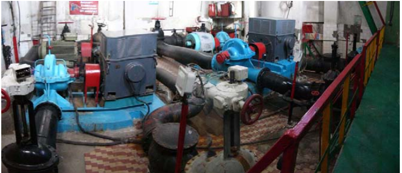
Overview of Pump Units in 2nd Station
