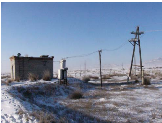
Pump House of 1st Station (2)
