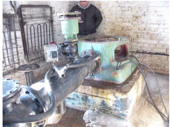
Inside of Pump House of 1st Station (1)
