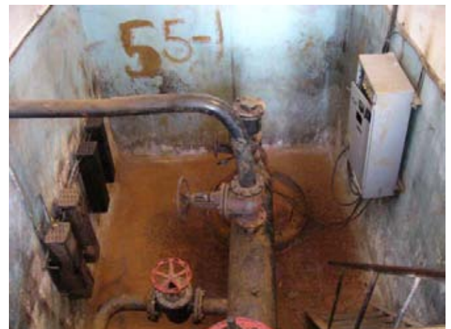
Inside of Pump House of 1st Station (2)
