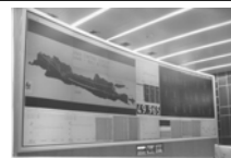
New SCADA at JCC in 2006
