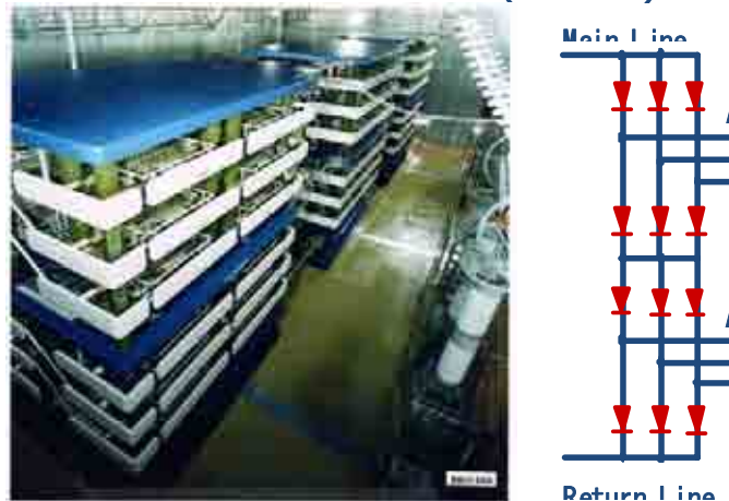
Fig.5.2-13 Compact Thyristor Valve installed in KIHOKU C/C (Key Equipment in C/C)
