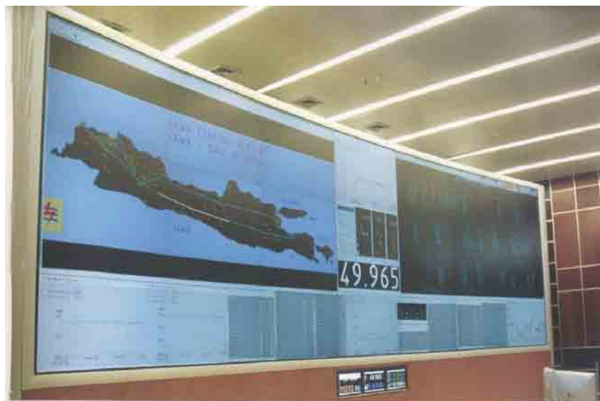
Fig.2.4-16 New SCADA of JCC
