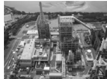
Demonstration Plant (250 MW) in Japan
