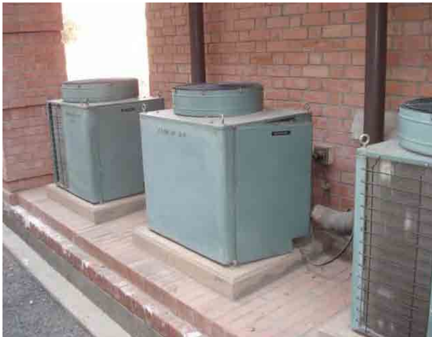
Cooling Units-Out of order
