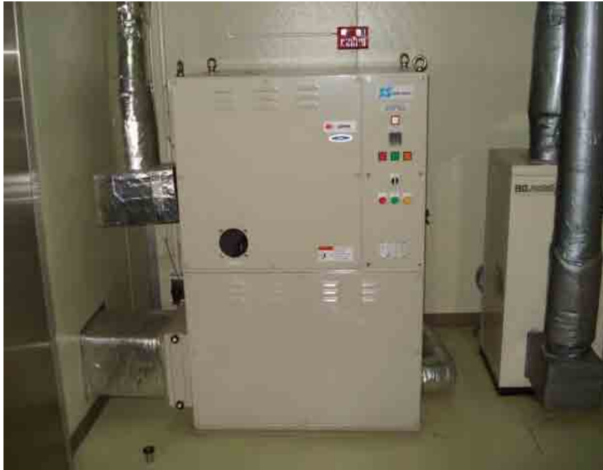
Dehumidifier Out of order
