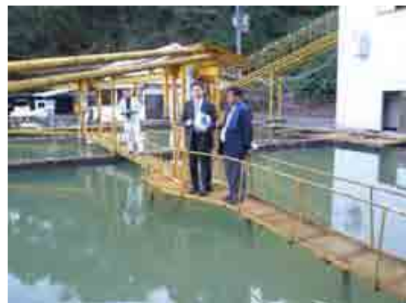
Photo 6.5.2 Myoho mine discharge water treatment plant
