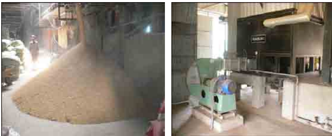
Figure 2.6-2 Rice Husk (left) and Co-generation System (Long An Province, AUSAID)
