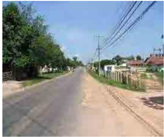
Collapsed Shoulder & Raveled Edge
