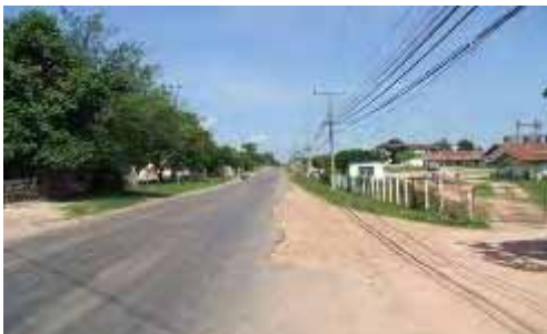
Collapsed Shoulder & Raveled Edge
