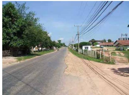
Collapsed Shoulder & Raveled Edge
