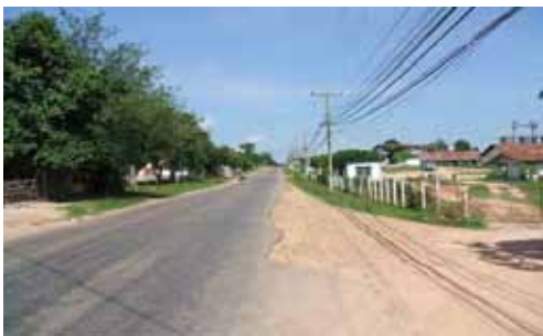
Collapsed Shoulder & Raveled Edge
