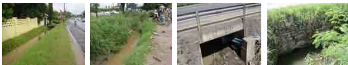
Figure 5.4.1 Drainage Facilities in New Bagamoyo Road
