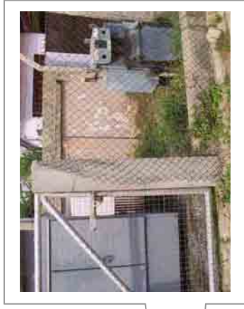
A242 Distribution transformer
