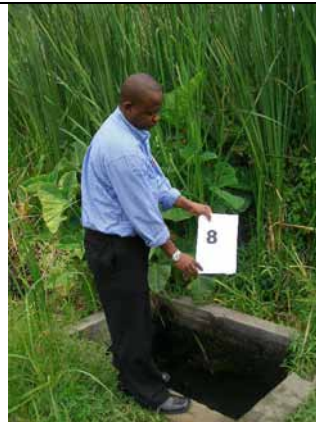
Point 8, Well, located at the foot of the road shoulder of Gerezani Road. Sometimes, local people use for washing agricultural tools and/or products. Remnant of floodplain bush exist.
