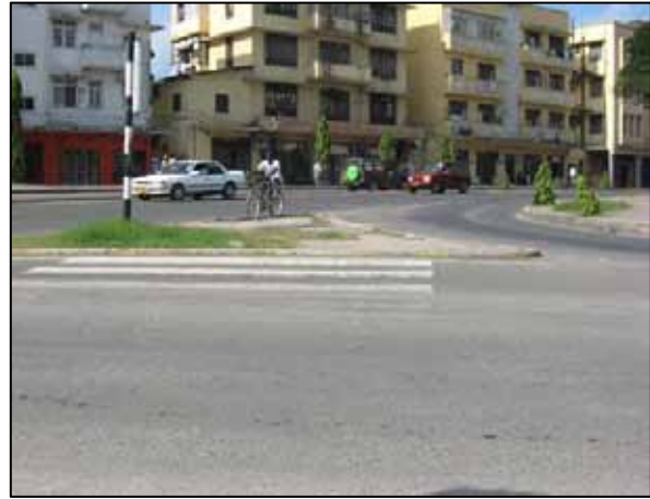
Figure 6.4.6 Worn Crosswalk Markings
