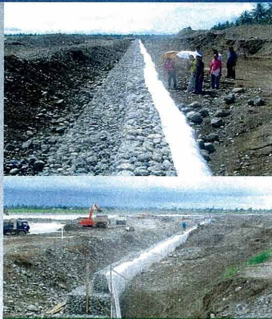
The Agos River re-channeling and gabion slope protection dike project in Infanta, Quezon with PHP 30 M fund from the national government. (Photo credit: Infanta MDCC)
