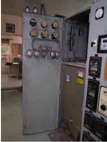
Internal condition of switchgear
