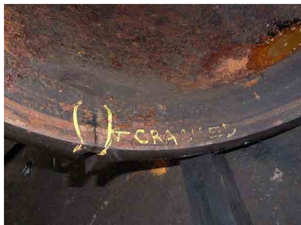
Cracking in the cooling water jacket
