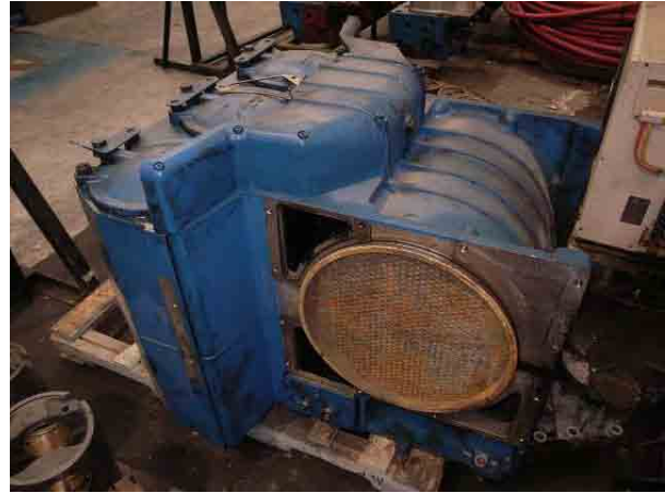
Lubricating oil cooler to be cleaned after opening
