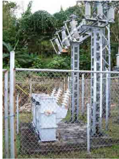
Fig. 2.4.2-13 Airai Substation (House-Service Transformer)
