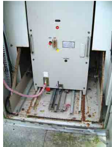
Fig. 2.4.2-17 Out-door Switchgear (inside)
