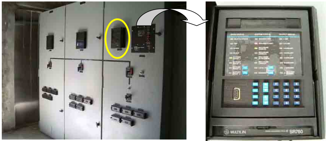
Fig. 2.4.2-23 Example of Protective Relay
