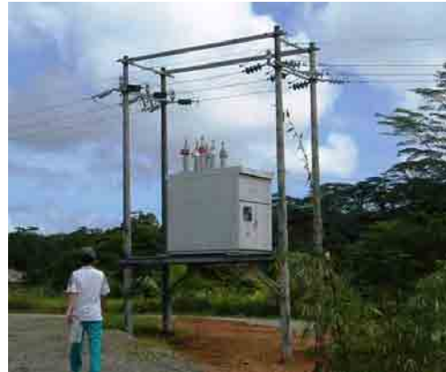
Fig. 2.4.2-2 Asahi Substation (circuit breaker for the transmission line)
