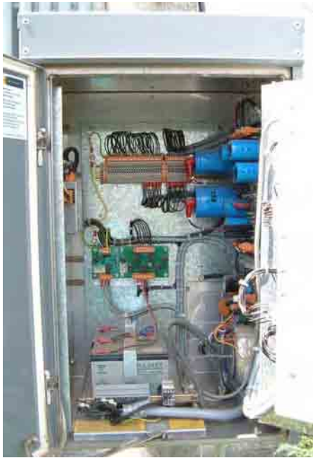
Fig. 2.4.2-11 Kokusai Substation (Recloser Control box)
