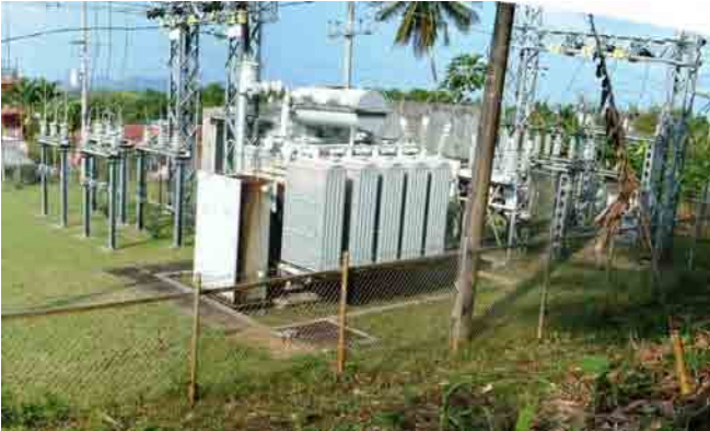
Fig. 2.4.2-8 Airai Substation (panoramic view)
