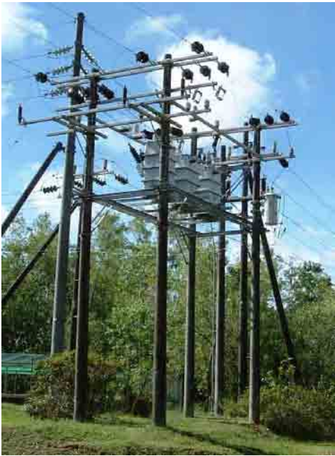
Fig. 2.4.2-10 Nekken Substation (panoramic view)
