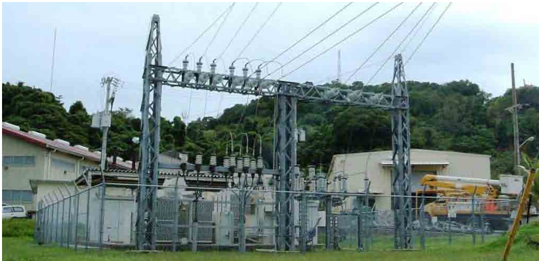
Fig. 2.4.2-7 Malakal Power Plant (transforming facilities)
