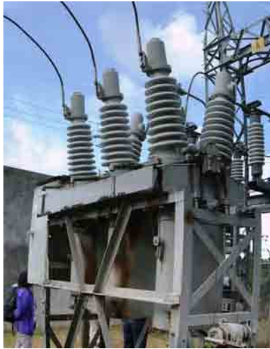
Fig. 2.4.2-12 Airai Substation (Oil Circuit Breaker)
