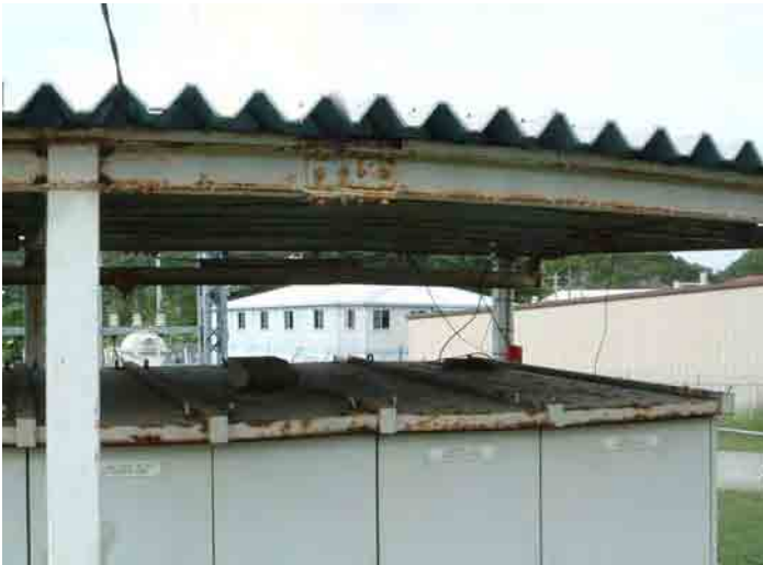
Fig. 2.4.2-16 Out-door Switchgear (outside)
