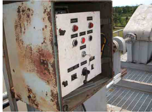
Control Panel is in working condition but heavily aged.
