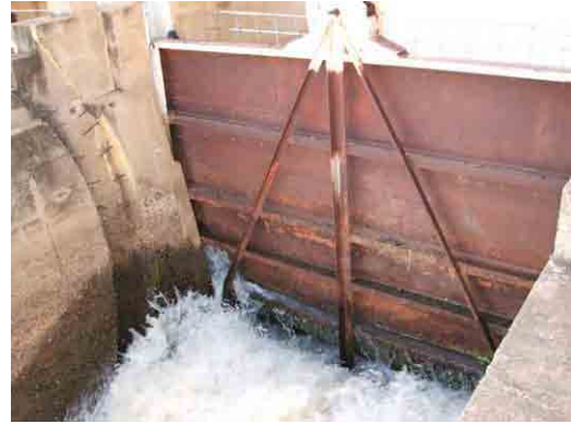
Corrosion and Leakage
