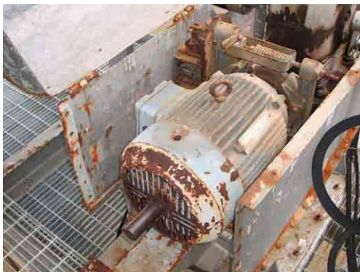
Electric Motor and Speed Reducer are in running condition, but heavily aged. Brake does not function.
