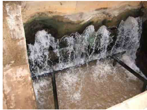
Leakage through Gate Top Seal
