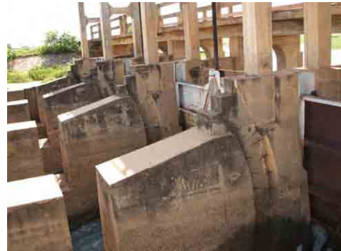
Box-out for side seal seat remains without filling concrete
