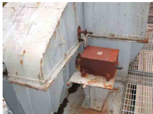
Limit Switch Box is broken.
