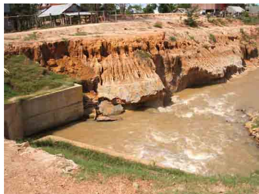
Severe Side Slope Erosion
