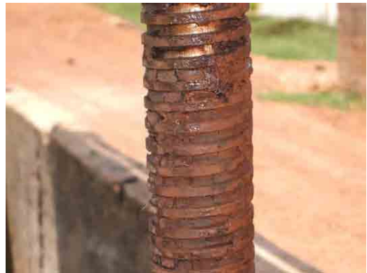
Debris in Spindle
