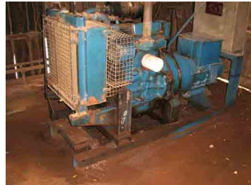
Diesel Generator is still working, but aged. No backup electric power source is available.
