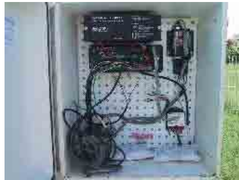
Data logger of rainfall, temperature etc. in box
