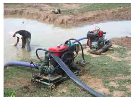
Types of portable pump used for taking water from the Prey Robong water harvesting reservoir
