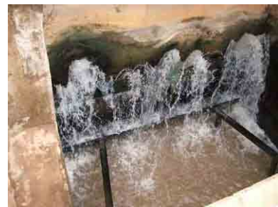
Leakage through Gate Top Seal Andong Sla Intake
