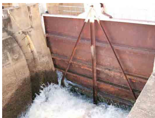
Corrosion and Leakage
