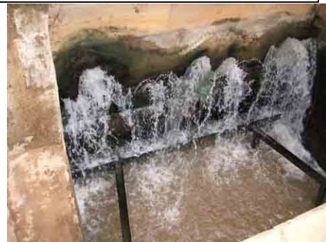
Leakage through Gate Top Seal
