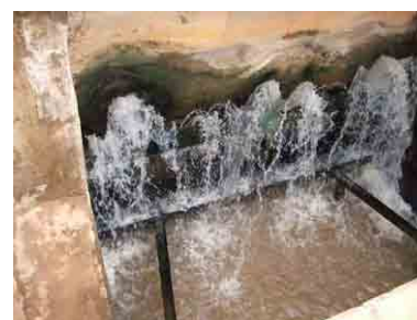
Leakage through Gate Top Seal Andong Sla Intake
