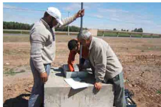
Setting up Automated Piezometers
