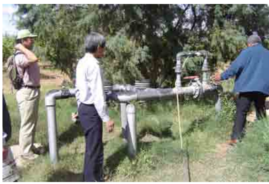
Filter System for Drip Irrigation
