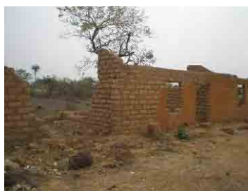
Wall Collapsed by Storm
