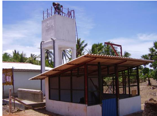
Construction of overhead tank for community water supply system by CMR (Theththavadi Maruthankulam)
