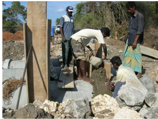
Construction of culvert incorporated with renovation of Attimodai-Kurai access road by CMR (Kurai)
