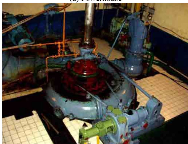
(b) Hydro Turbine
