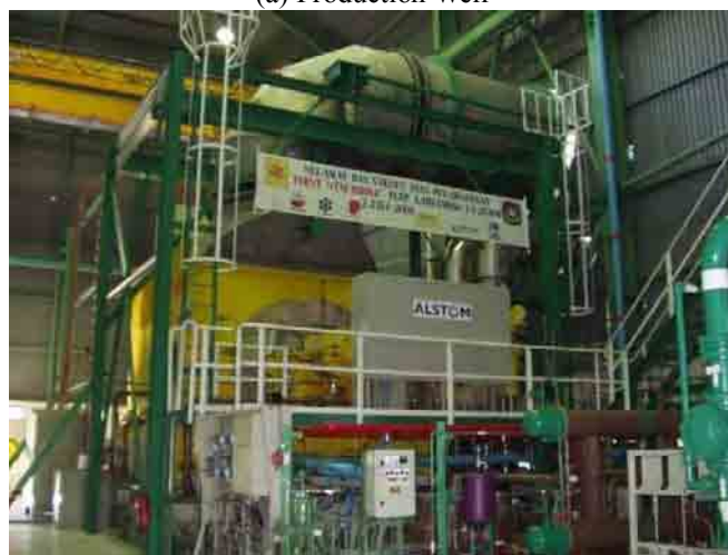
(b) Geothermal Plant
