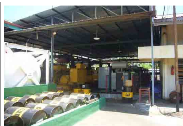
Figure 5.4.1 Gorontalo Diesel Power Plant
